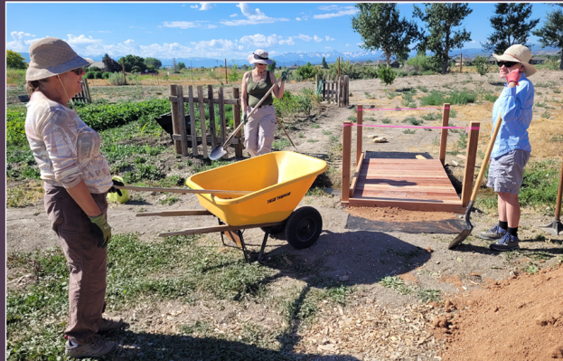
Debby Ingram, Peggy Justis and Liz Mauch appreciate the new bridge across the Homestead Garden's irrigation ditch, which was built by MBS member Tim Garvey.
