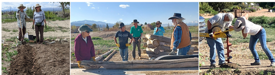
Planting row crops; assembling the logs of the historic cabin from Cerise Park; and digging postholes for interpretive signs.
